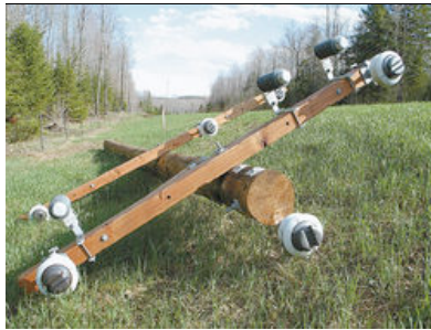
Power poles are lying alongside Marquette County Road 550, ready to be installed as part of an electric system upgrade project currently ongoing by the Alger-Delta Cooperative Electric Association. The new lines are expected to be energized in July. (Journal photo by John Pepin)
